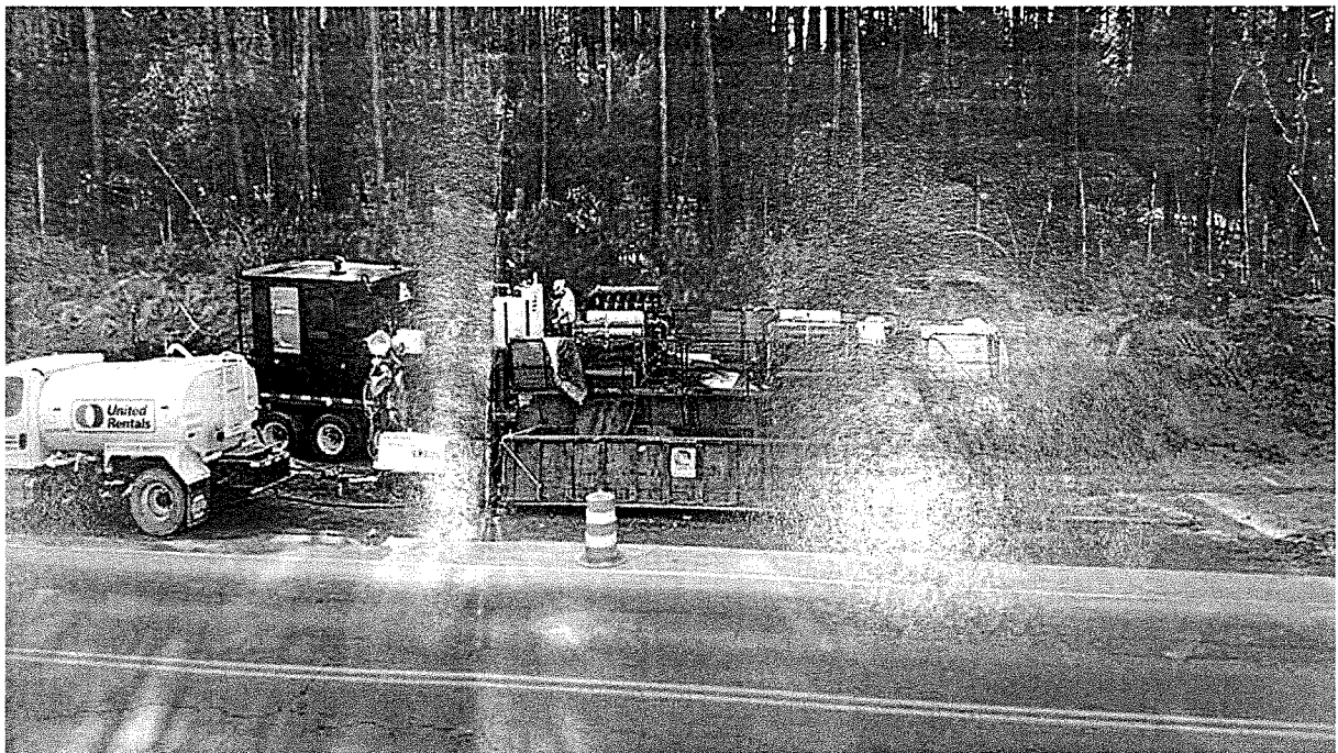
Photo 5 - Shaker and Roll-Off Bin (Front View)
