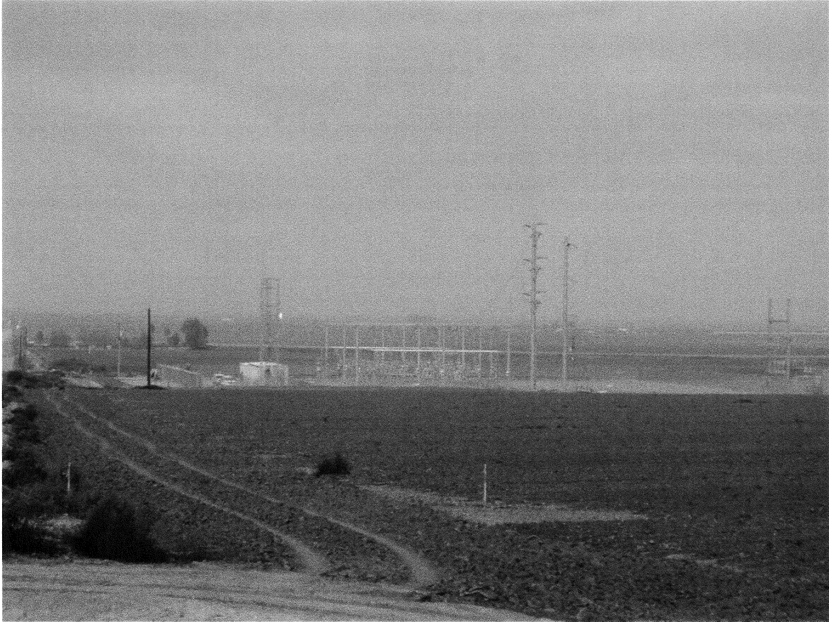
Photo 1. Typical 70 kV switching station.
