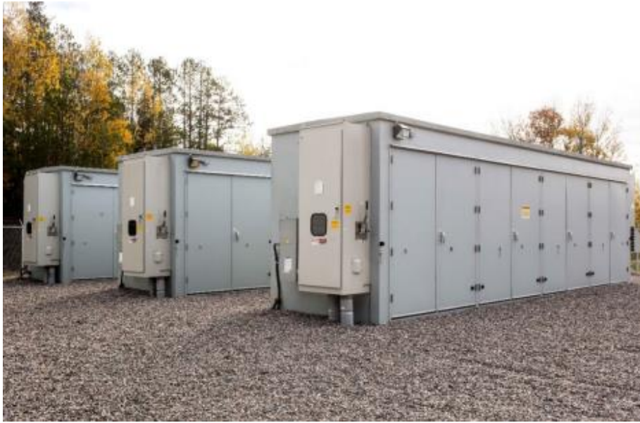
Figure 3 Examples of Energy Storage Units
