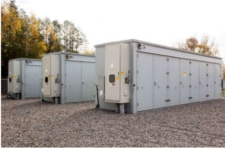
Figure 1 Examples of Energy Storage Units
