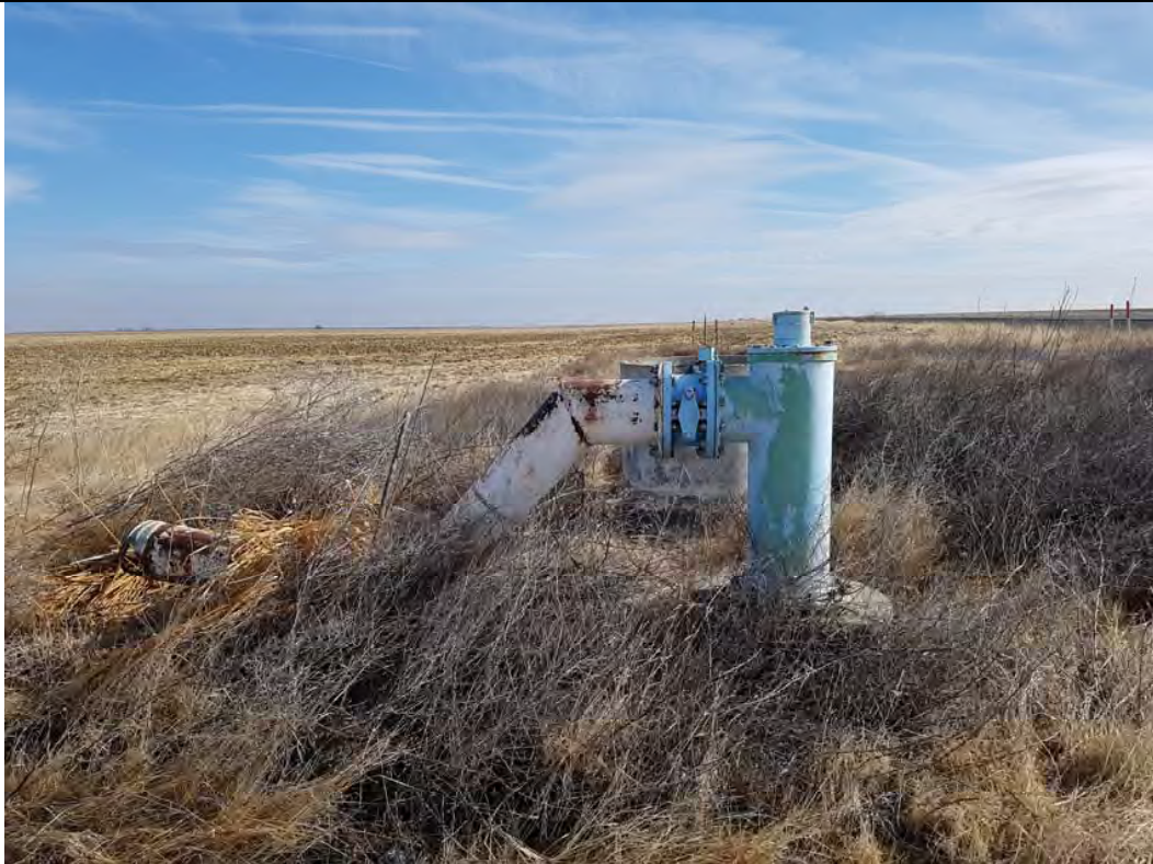
Photograph: 13 View of irrigation piping access/pump location, located in the central western portion of the Site.
