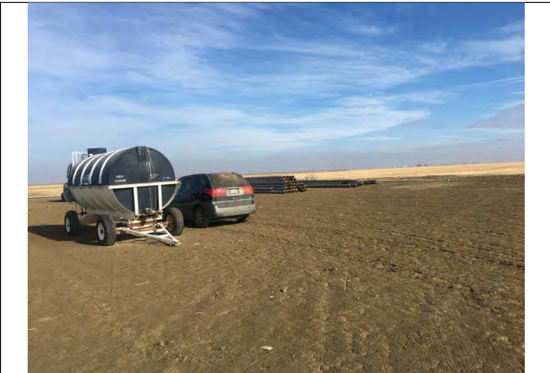
Photograph: 2 | View of portable water tank and piping for the adjacent site irrigation development located in the northwestern corner of the Site.
