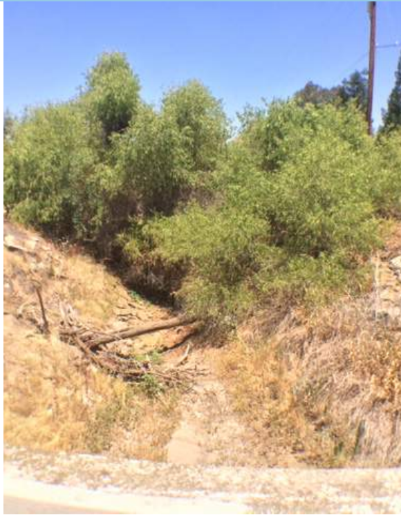
Photo #1. Travers Creek, north of the existing bridge (photo taken on top of bridge).
