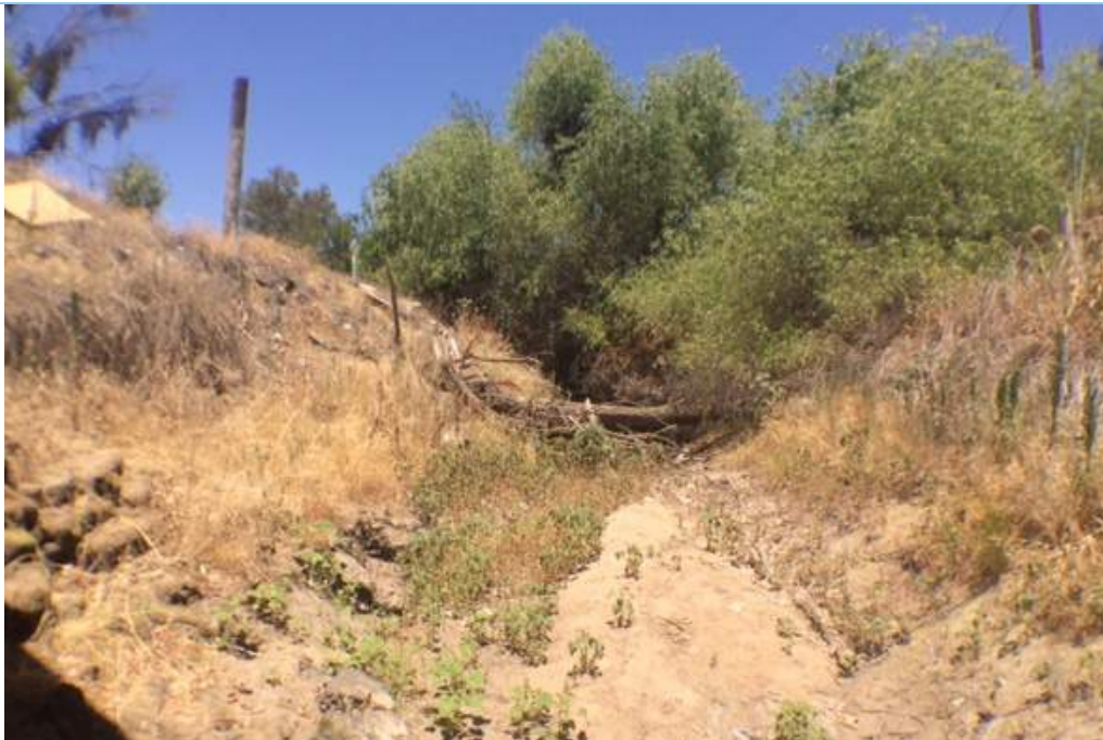
Photo #6. Travers Creek, north of the existing bridge (photo taken beneath the bridge).
