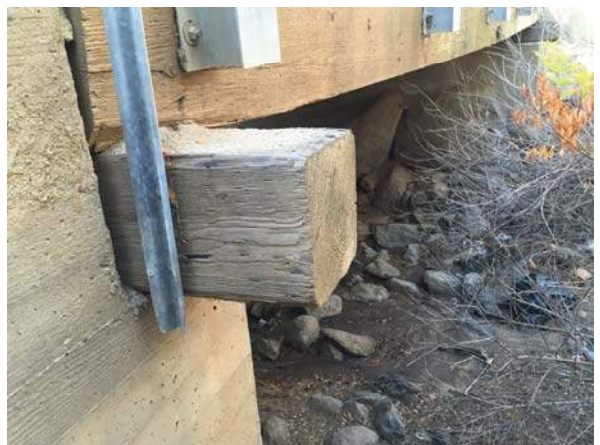
Photo #6 View of beneath the south side of Sand Creek Bridge, facing northeast.
