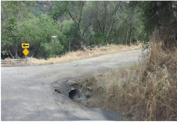
Photo #7 Existing storm drain under Hummingbird Lane (West approach of Sand Creek Bridge and Hummingbird Lane).
