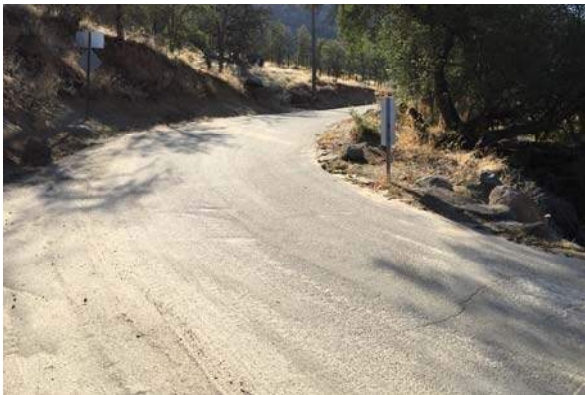
Photo #3 View of Ennis Road east of Sand Creek Bridge, facing east.
