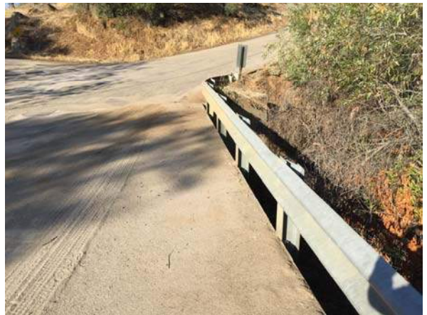
Photo #4 View of the north side of Sand Creek Bridge, facing southwest.
