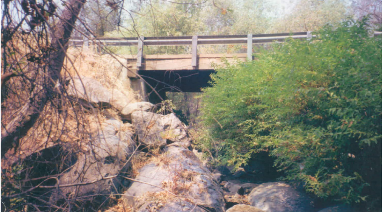
Figure 5. Looking upstream at the channel. The creek bottom is heavily vegetated and the bank and overbank areas are vegetated with higher manning “n” values.
