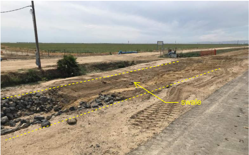
Figure 11 Additional drainage swale illustrating a shallow depression at the Outside Canal Bridge Replacement Project on Russell Avenue.
