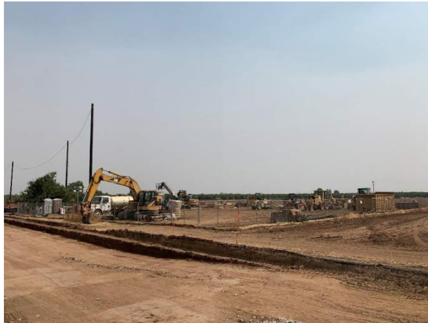
Figure 4 Temporary construction yard during construction. Fresno Canal Bridge Replacement Project on McKinley (current project).
