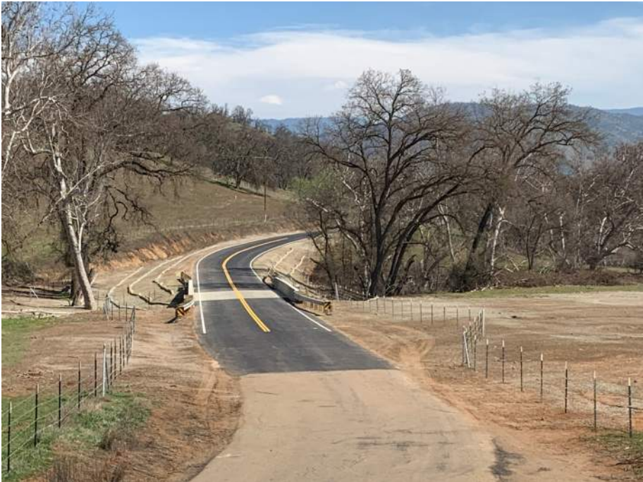
Figure 12 View of the completed bridge and project site at Watts Creek on Watts Valley Road.
