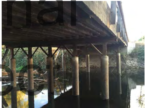
Photo #4 View of the underside of the Fresno Canal Bridge, facing south.
