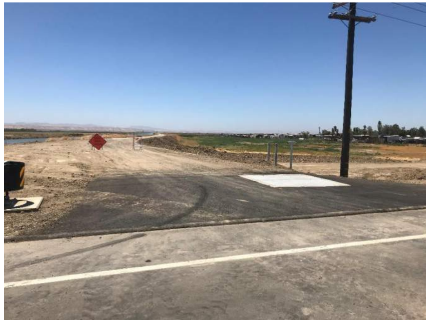
Figure 5 A realigned access road with paved driveway at the Outside Canal Bridge Replacement Project on Russell Avenue.
