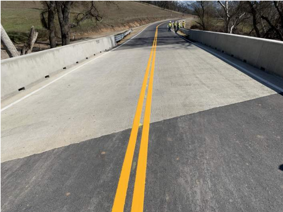
Figure 13 View of the top of completed bridge and project site at Watts Creek on Watts Valley Road.
