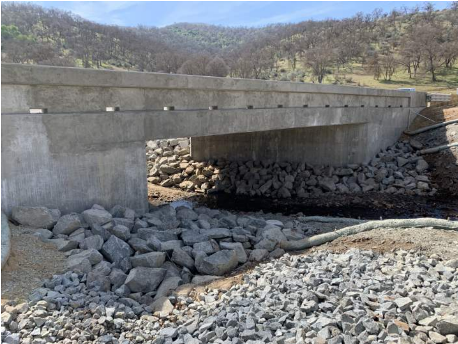
Figure 14 Side view of the completed bridge and project site at Watts Creek on Watts Valley Road.
