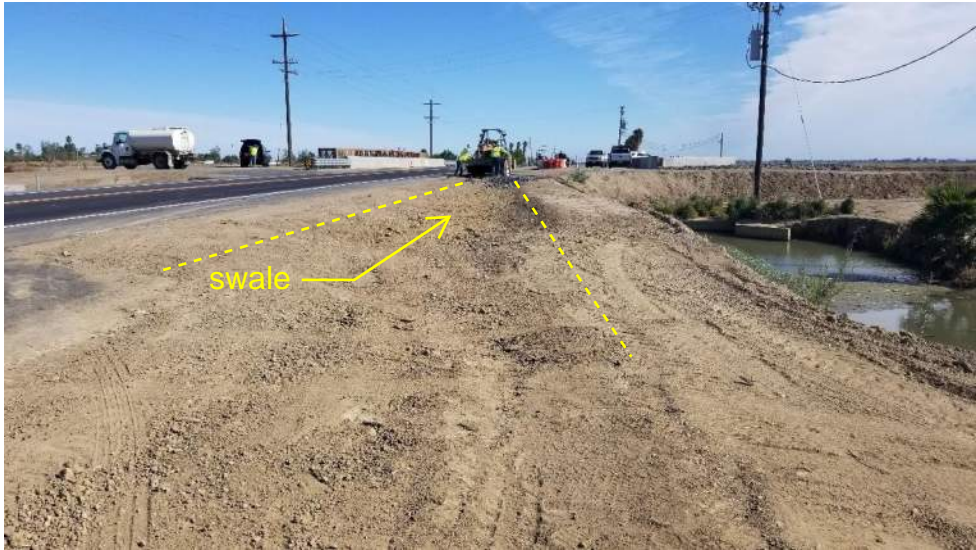
Figure 9 Graded drainage swale next to a small drainage canal at the Outside Canal Bridge Replacement Project on Russell Avenue.
