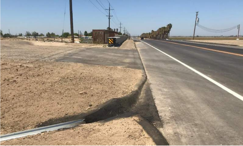
Figure 6 An additional realigned access road with a paved driveway at the Outside Canal Bridge Replacement Project on Russell Avenue.
