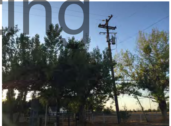
Photo #6 View of an electrical transformer north of the Fresno Canal Bridge and west of N. Del Rey Avenue, facing northwest.
