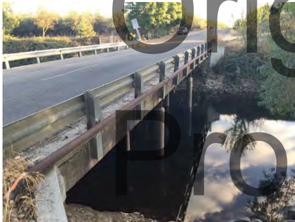
Photo #3 View of the west side of the Fresno Canal Bridge, facing south.
