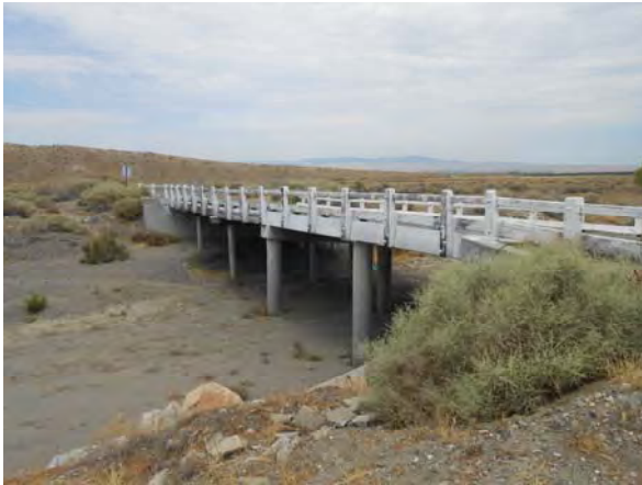
Photo #1 View of Jacalitos Creek Bridge and Lost Hills Road, facing north.
