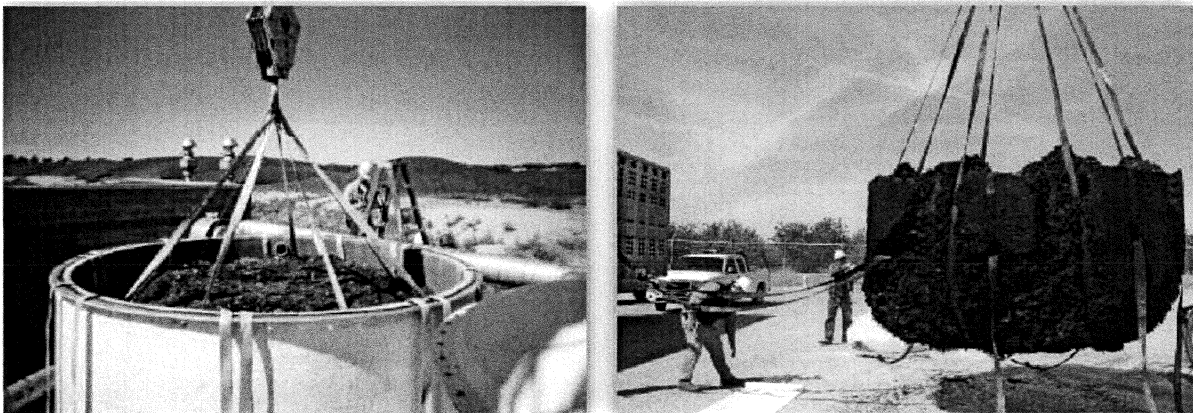
Figure 8 -- MV Tech H 2 S Scrubber
