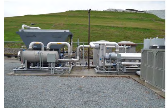
Picture 2 – Chiller & Dryer Skid
