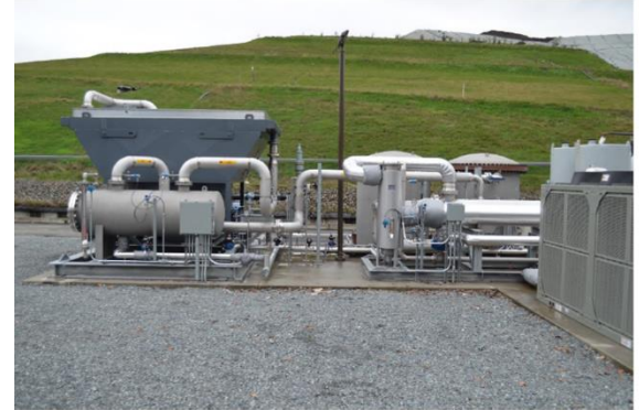
Picture 2 – Chiller & Dryer Skid
